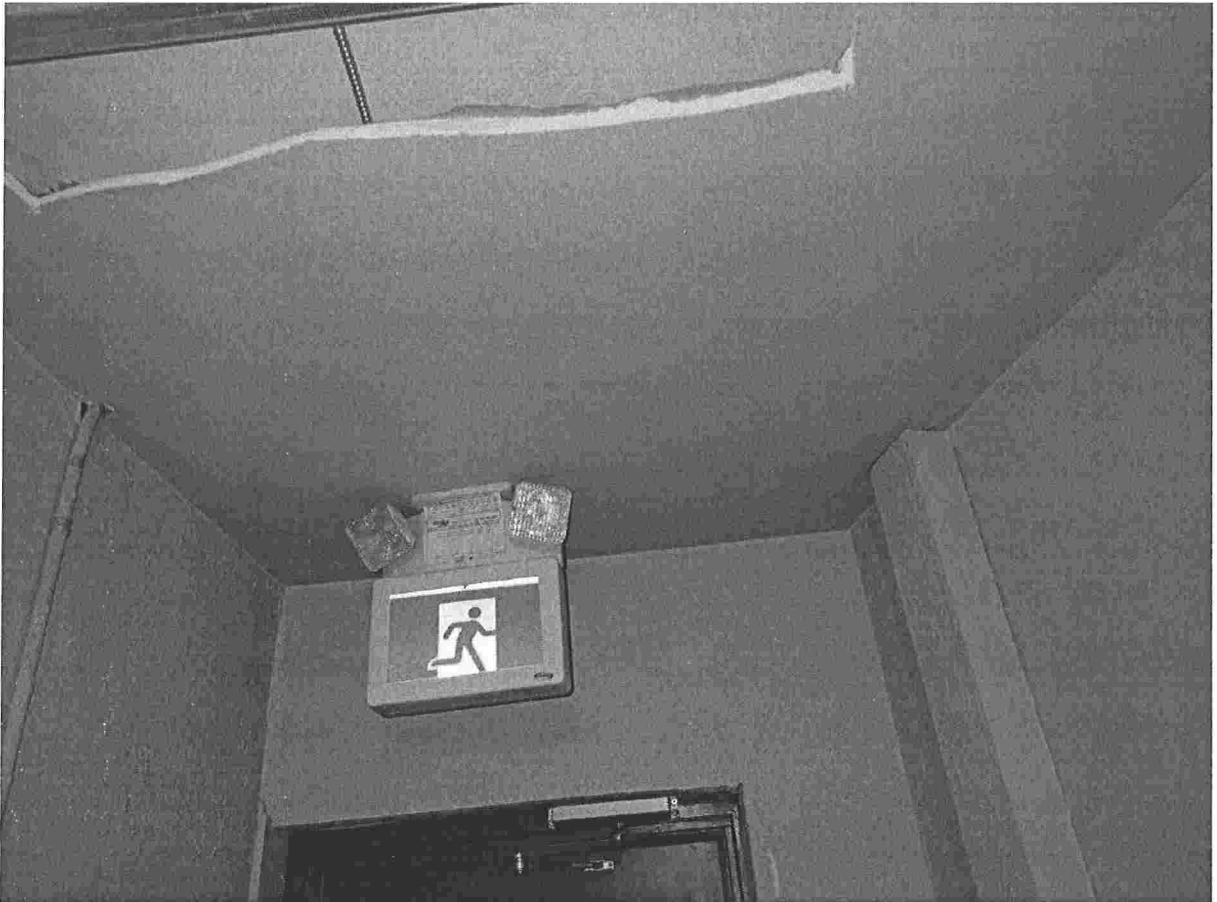
Photo 12 – Level 1 typical combination exit/emergency lighting
