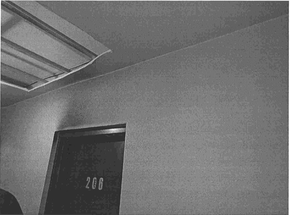
Photo 14 – Some soot exiting Unit 206
