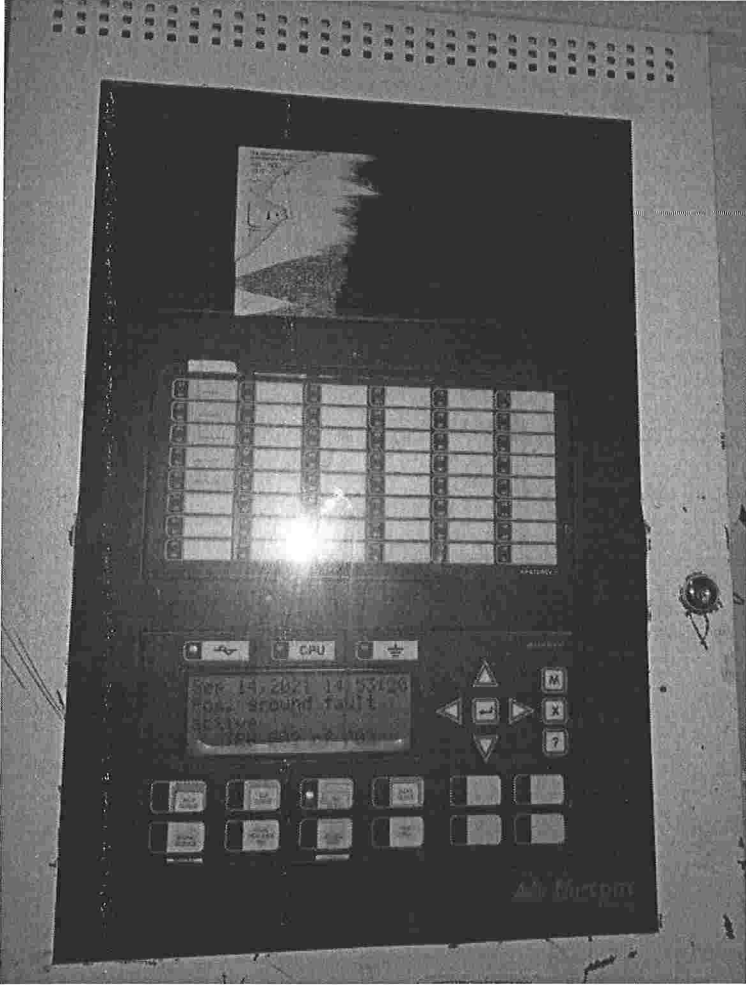
Photo 18 – Main fire alarm panel at main entrance
