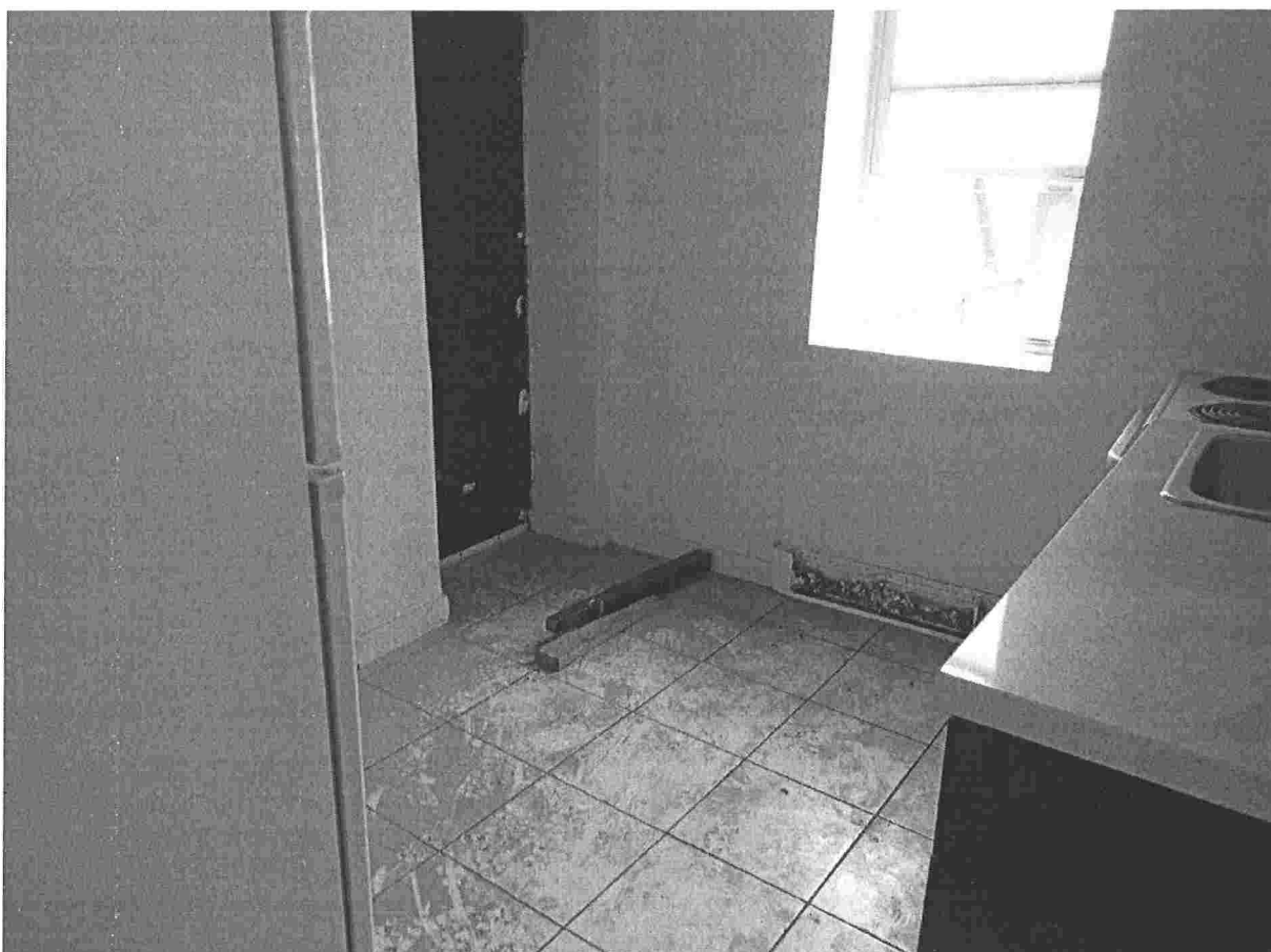
Photo 17 - Unit 306 – Soot from fire damaged Unit 206 below.
