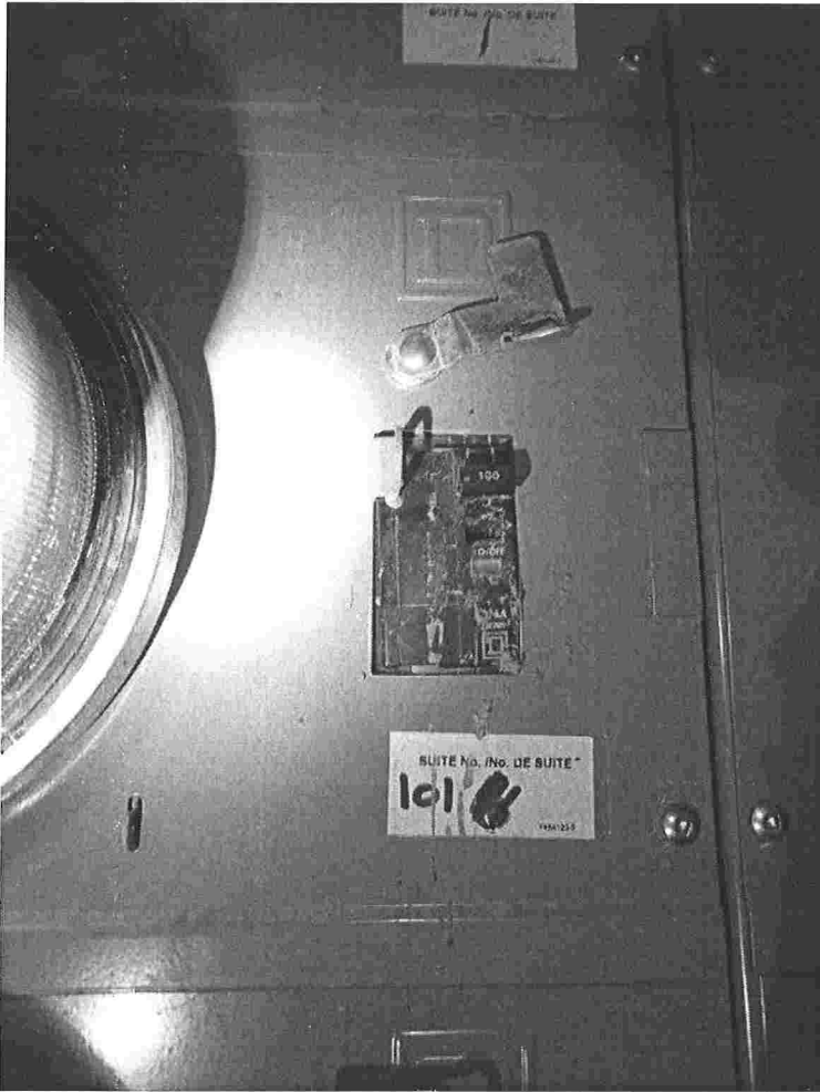
Photo 3 – Close up of water damage to meter centre .
