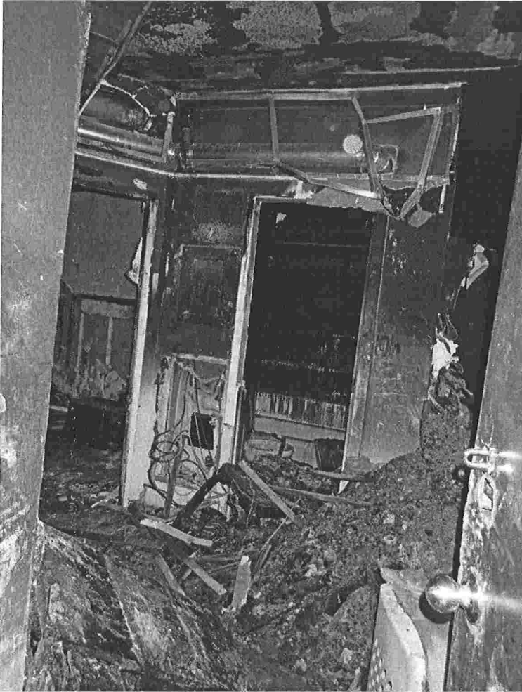
Photo 13 – Fire damaged suite (Unit 206)
