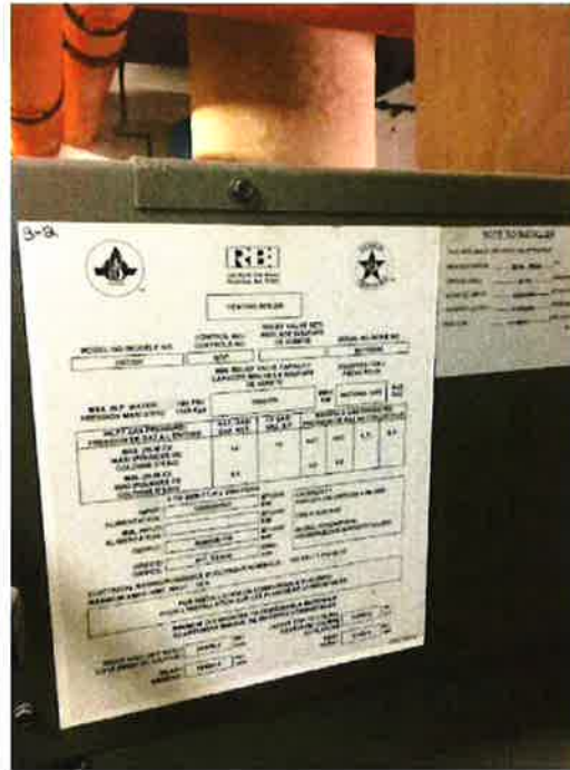
Photo 16: Typical RBI natural gas heating boiler tag, estimated age to be 2008
