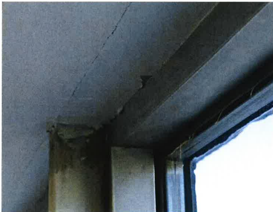
Photo 16: Loose glazing stop on 10 th floor level
