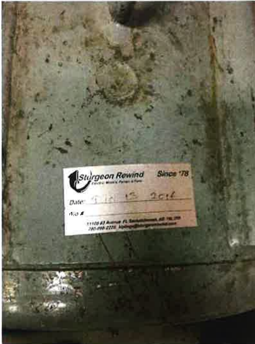
Photo 27: AHU fan motor serviced in 2016
