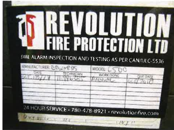
Photo 17: Fire alarm control panel annual testing
