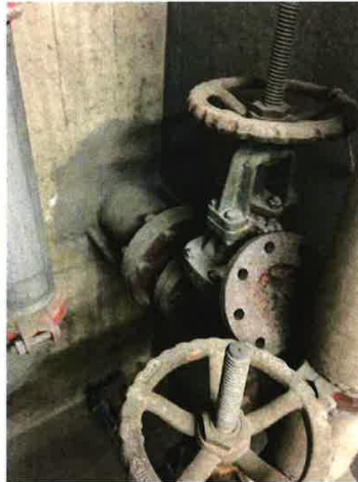
Photo 88: Incoming domestic cold water service, flanged pipe shows signs of a previous blockage
