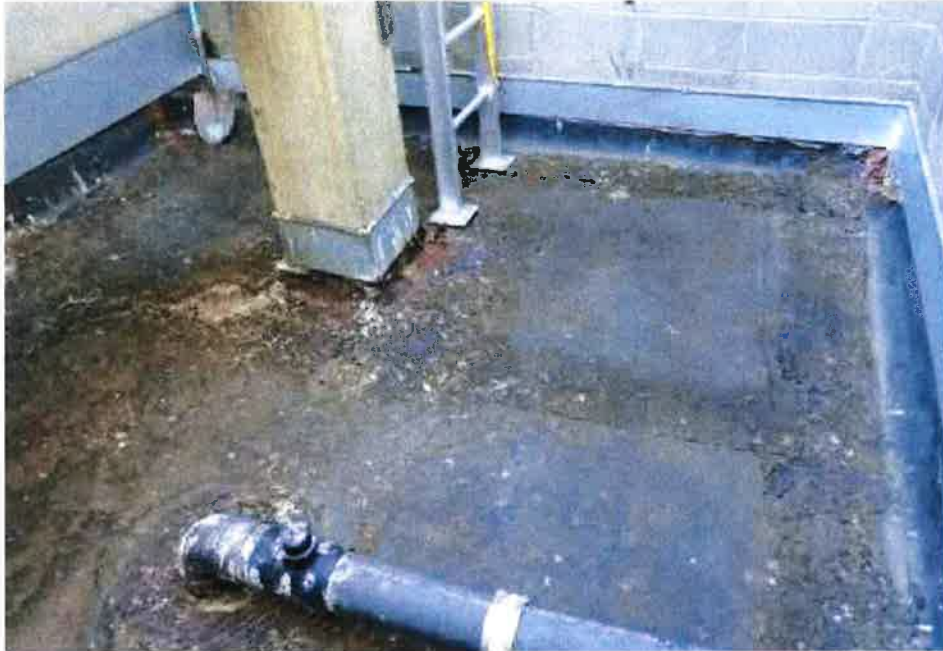
Photo 13: Deteriorated roofing below Cooling Tower
