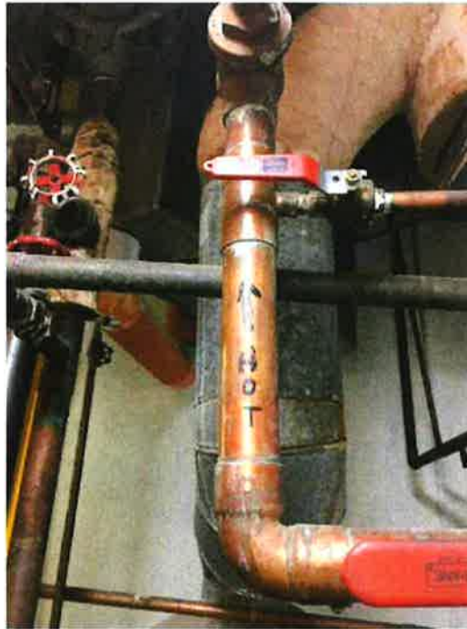
Photo 9: Uninsulated domestic hot water piping
