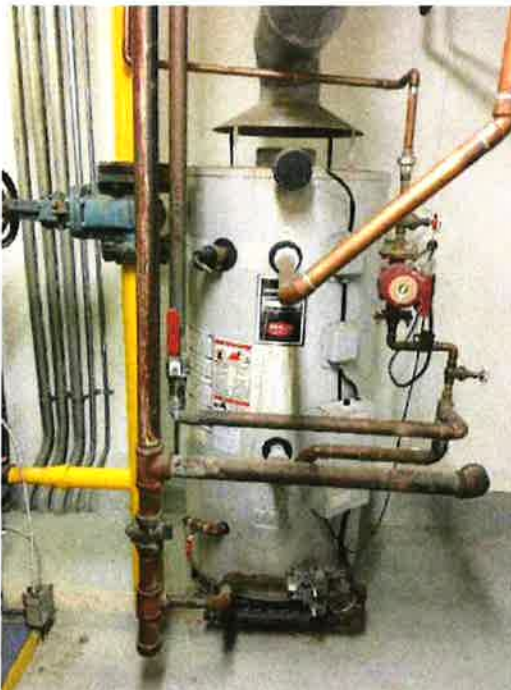
Photo 7: Natural gas fired, 246 litre (65 gallon), 22.6 L/min (6 gpm) recovery, domestic hot water tank
