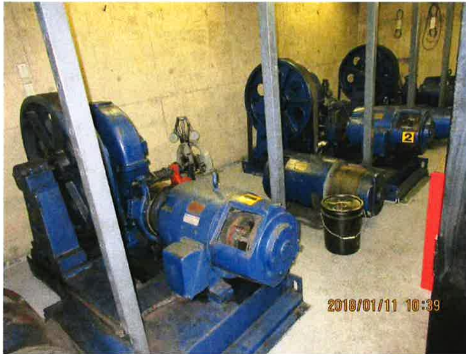
Photo 1: Geared hoist machines (Passenger 1-3)
