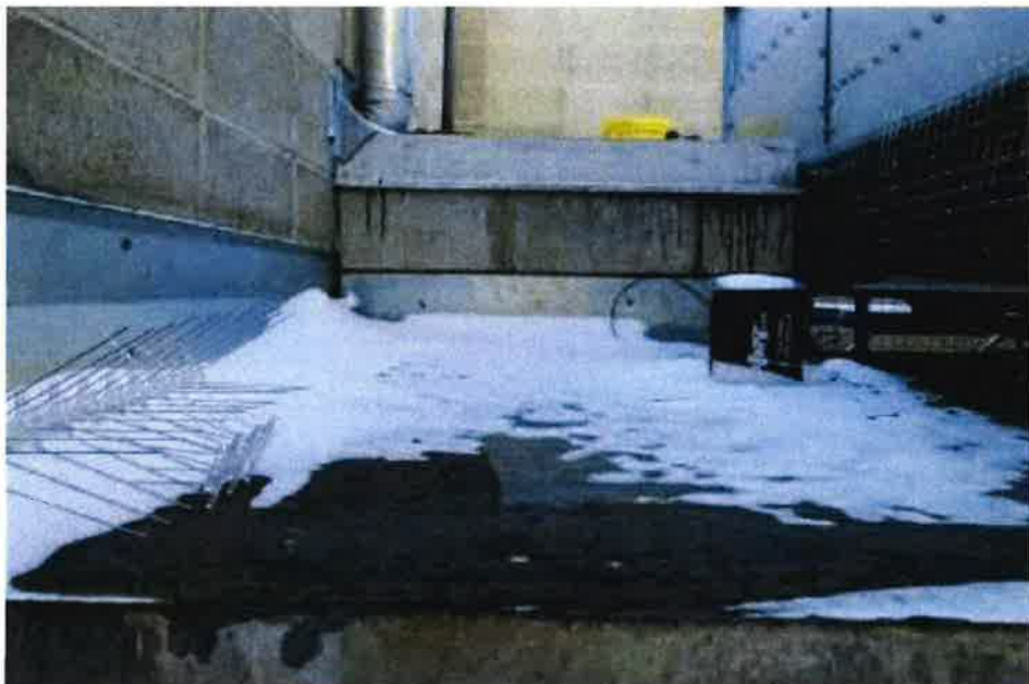
Photo 12: Deteriorated roofing near Cooling Tower
