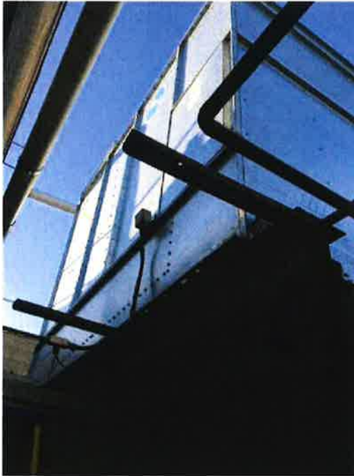
Photo 62: Cooling tower from below
