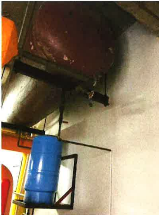
Photo 19: Heating system expansion tanks
