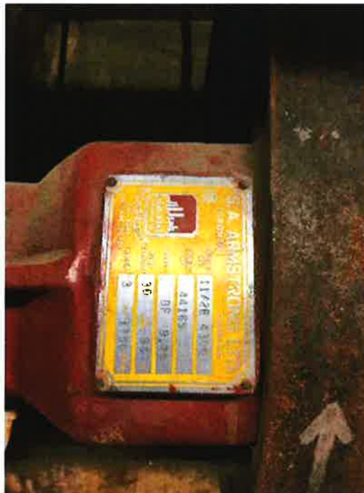
Photo 104: Glycol pump tag
