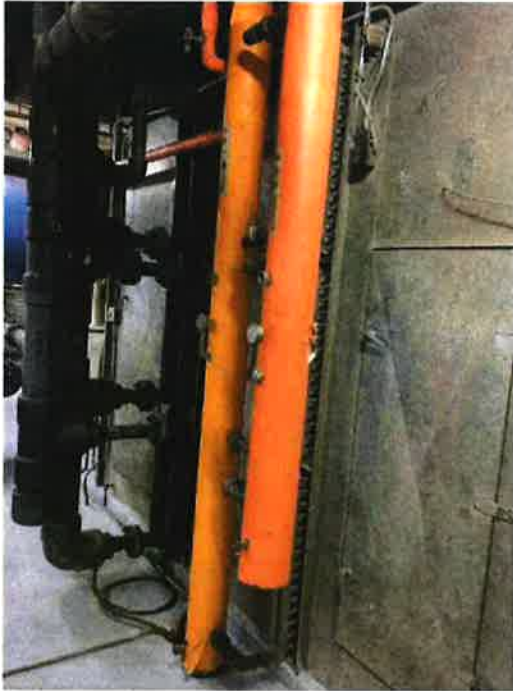
Photo 51: AHU1 hot water and cooling coil
