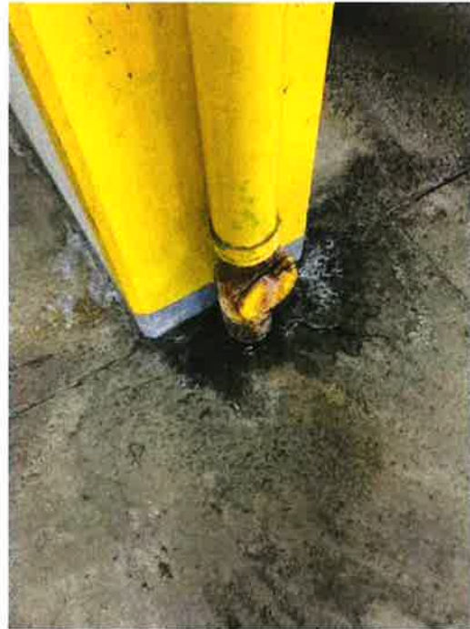
Photo 116: Drainage piping, cleanout cover not closed properly showing signs of corrosion
