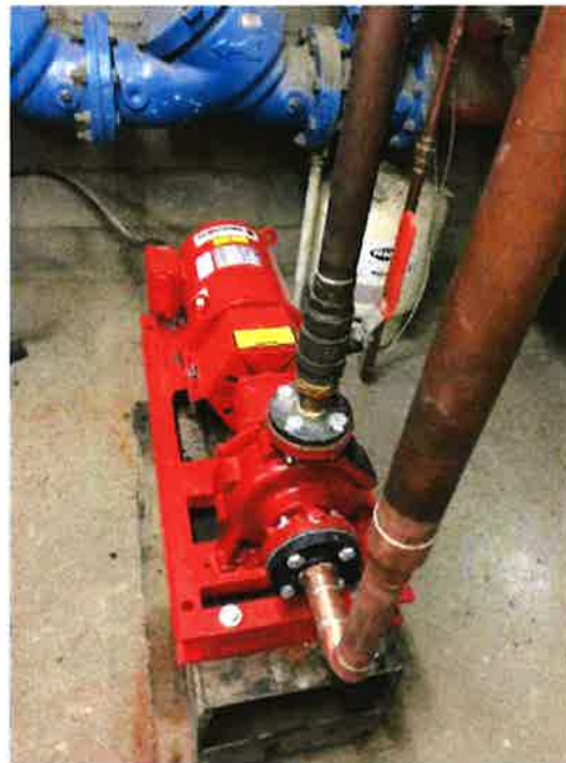
Photo 90: Primary domestic cold water booster pump
