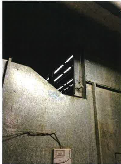
Photo 67: Intake louvre to mechanical room
