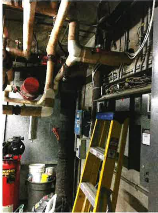
Photo 109: Glycol loop piping
