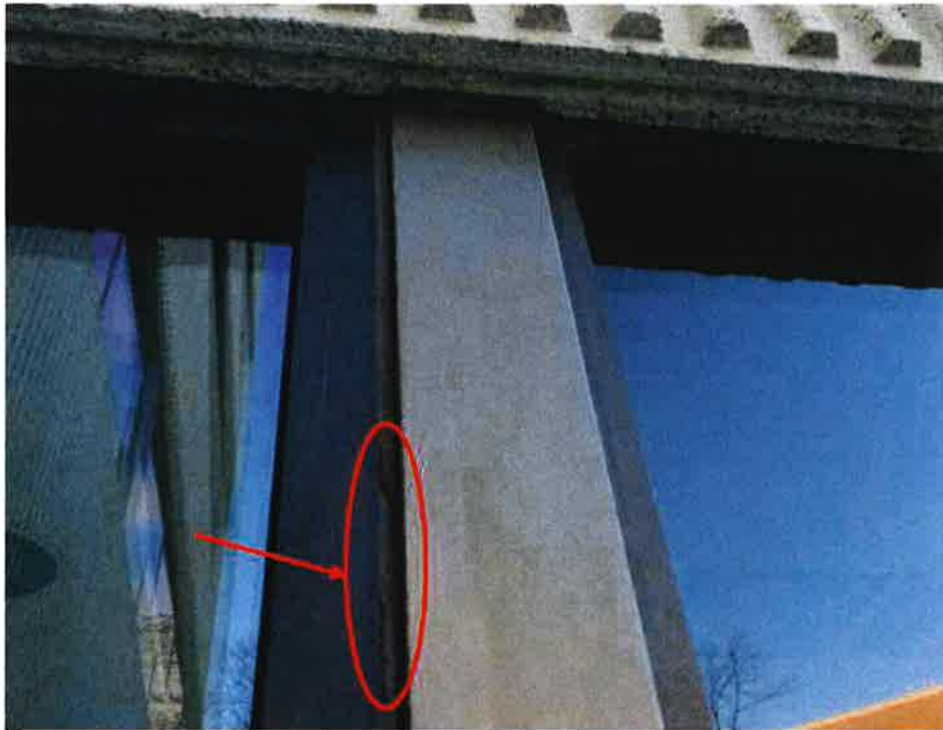
Photo 13: Failed caulking between aluminum frame and metal panel
