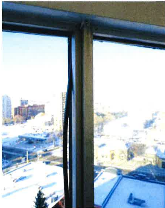
Photo 15: Loose interior gasket on 10 th floor window
