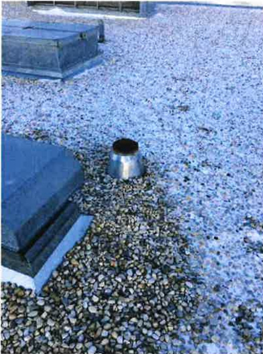
Photo 123: Roof - termination, not high enough off roof
