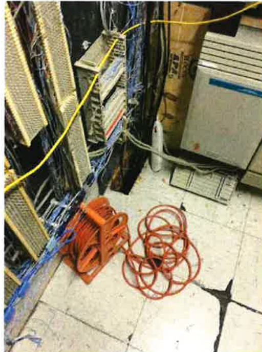
Photo 69: Typical electrical room floor, missing fire stopping
