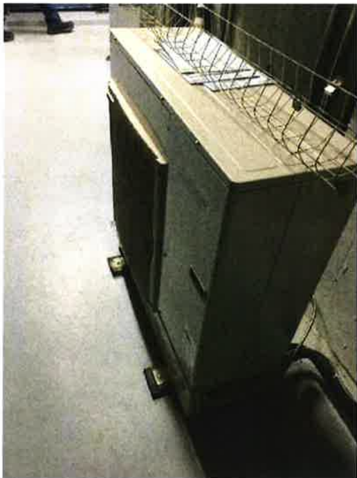
Photo 45: Condenser for spit air conditioning system
