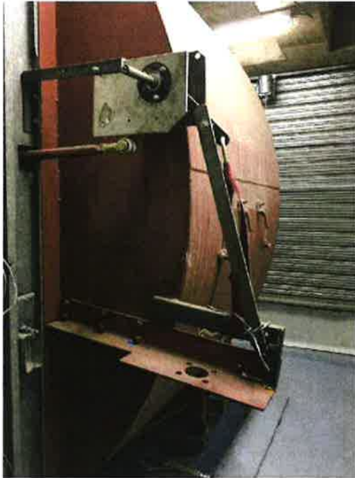
Photo 59: AHU1 damper, actuator motor is missing, wired into position
