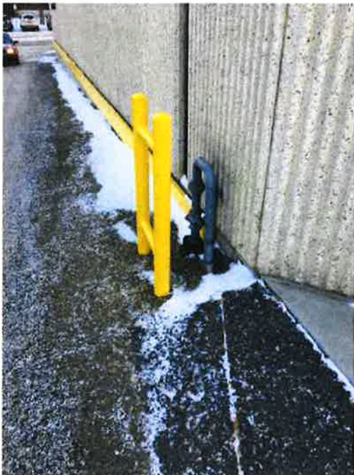
Photo 125: Gas shut-off outside of building
