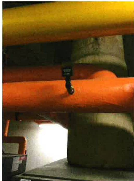
Photo 22: Digital temperature gauge on heating line
