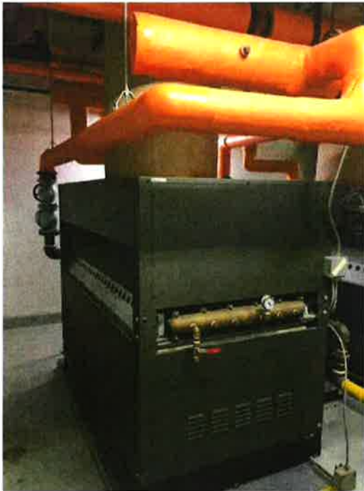
Photo 15: RBI natural gas heating boiler
