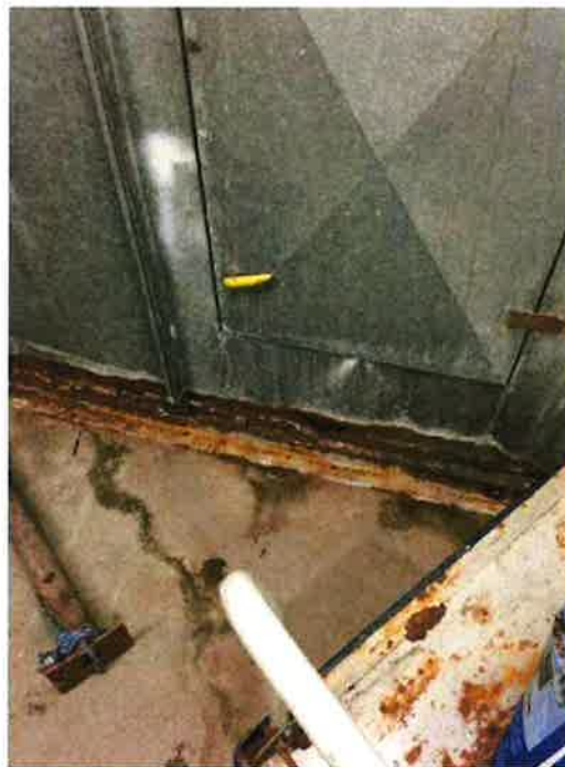
Photo 100: Parkade exhaust fan air plenum up to first floor roof, showing water damage
