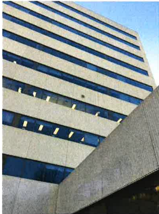
Photo 128: Louvre at front of building
