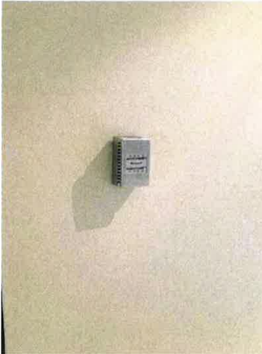
Photo 5: Typical pneumatic thermostat
