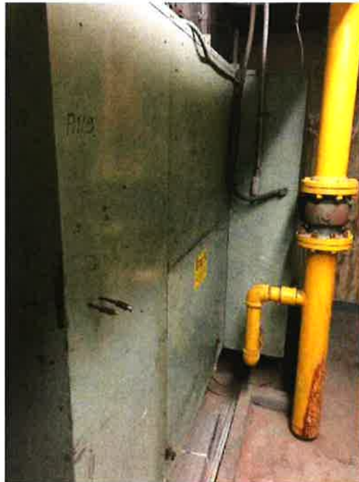
Photo 83: Make-up air unit (MAU) for parkade ventilation
