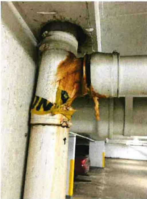
Photo 117: Drainage piping, showing fitting in poor condition
