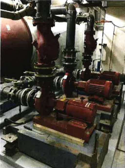
Photo 53: Chilled water pumps
