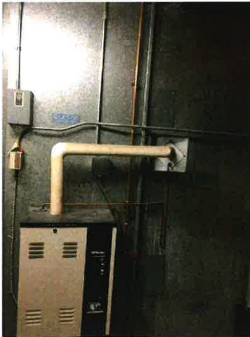
Photo 29: 30.6 kW Humidifier 'H2', servicing AHU2
