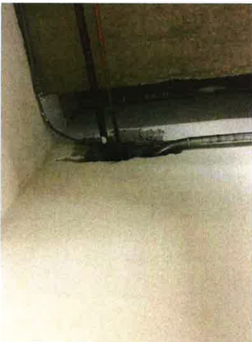
Photo 13: Fire stopping missing at mechanical room wall
