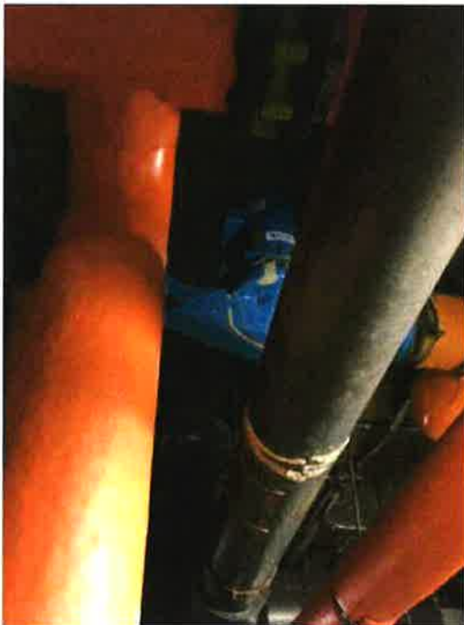
Photo 41: AHU2 heating coil pump
