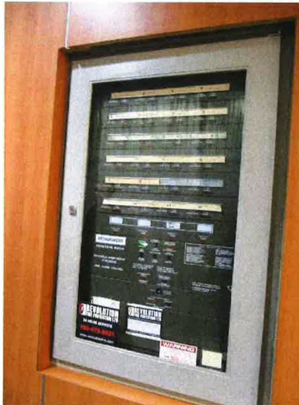
Photo 15: Fire alarm control panel
