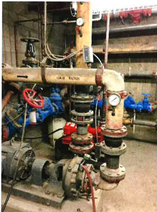
Photo 95: Domestic cold water piping with booster pumps, fire protection DCVA and domestic DCVA in background
