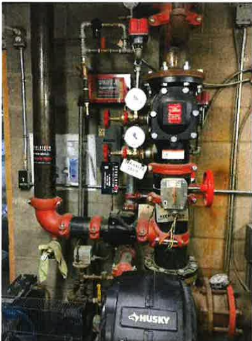
Photo 97: Sprinkler tree, showing supervised valve wires not connected. Valve is chained off.
