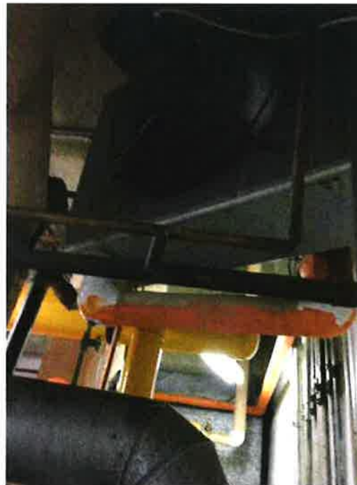
Photo 12: Hydronic unit heater in mechanical room
