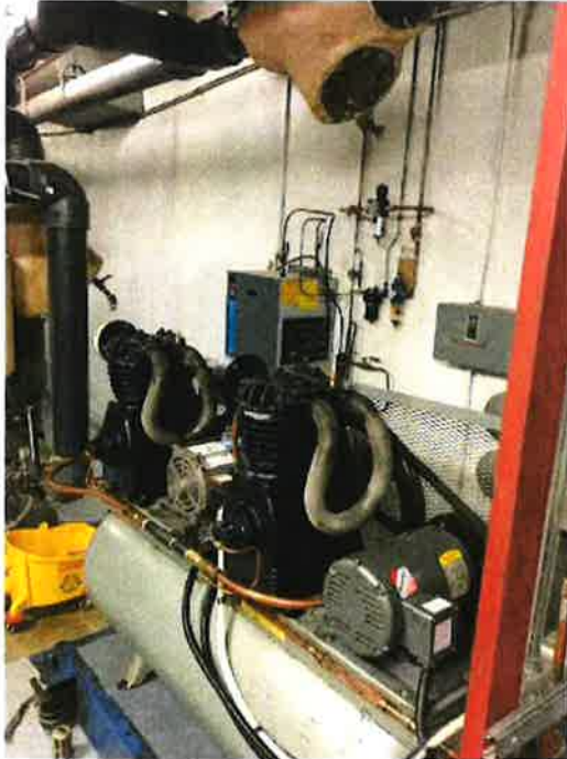
Photo 39: Air compressor and air dryer for pneumatic controls
