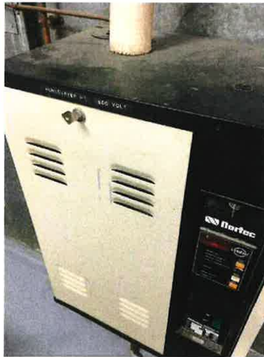
Photo 56: Humidifier 'H1' for AHU1
