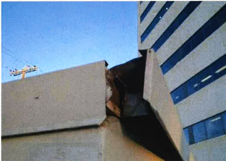
Photo 14: Damage at corner of mechanical doghouse roof
