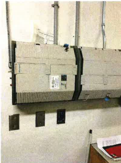
Photo 21: Air handler control panel
