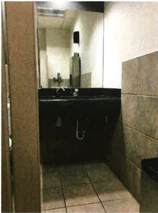
Photo 1: Typical washroom vanity with automatic hands-free sink
