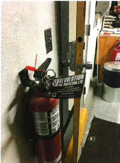
Photo 11: Fire extinguisher inside mechanical room
