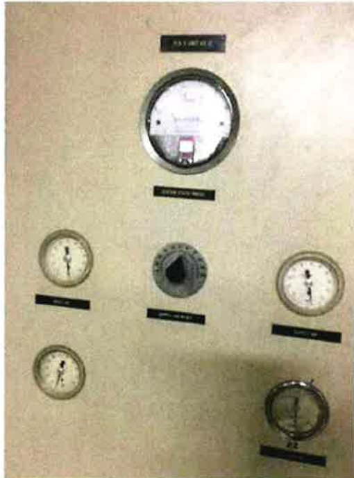
Photo 37: Honeywell control panel for AHU2 (Control CCT 33, Panel A) Part 2
