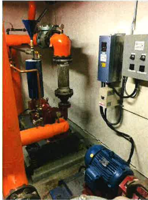
Photo 24: Lead and lag heating pumps. Lead pump is on VFD controller.
