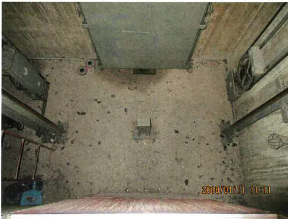
Photo 6: Typical pit area (Passenger 1-3)
