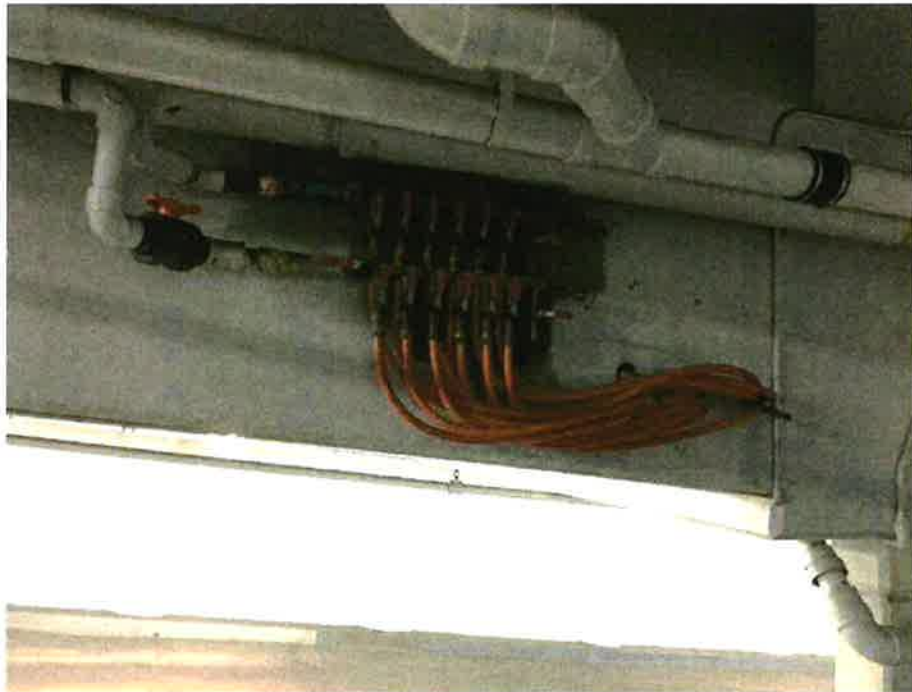
Photo 110: Parkade ramp glycol manifold and slab piping
