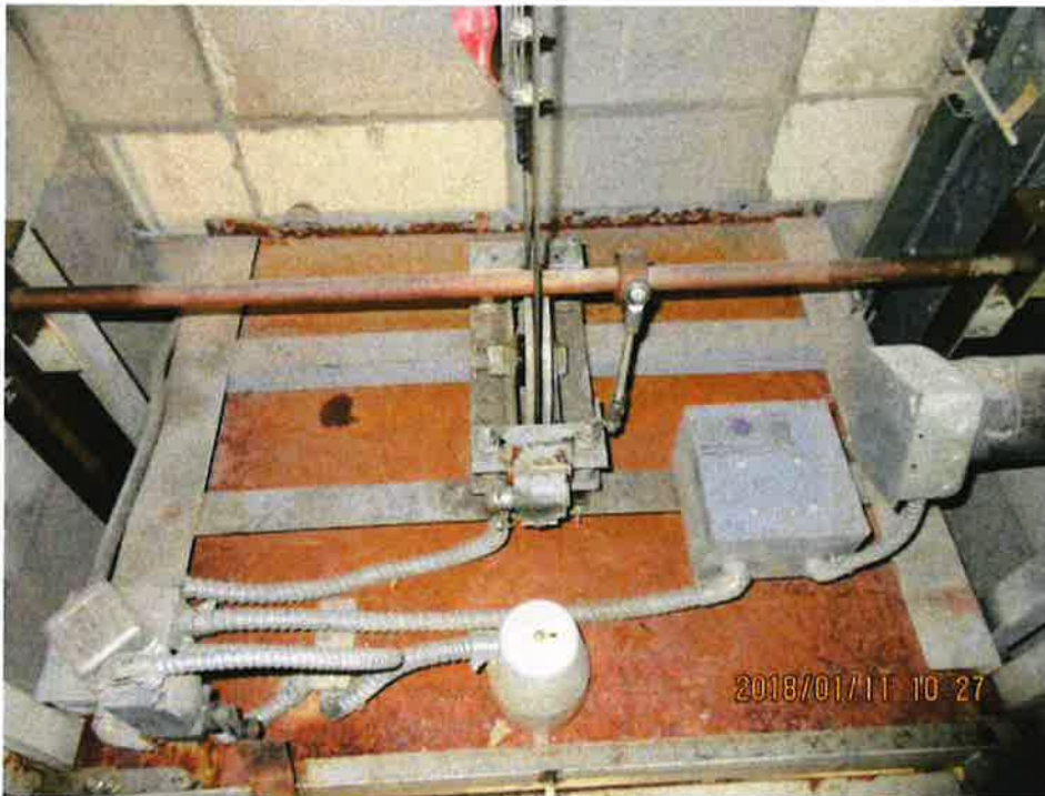
Photo 20: Car top area (Dumbwaiter 5)
