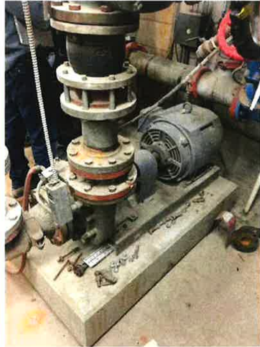
Photo 92: Domestic cold water booster pump
