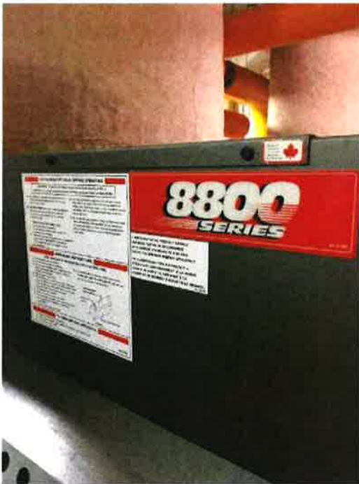
Photo 17: RBI natural gas heating boiler
