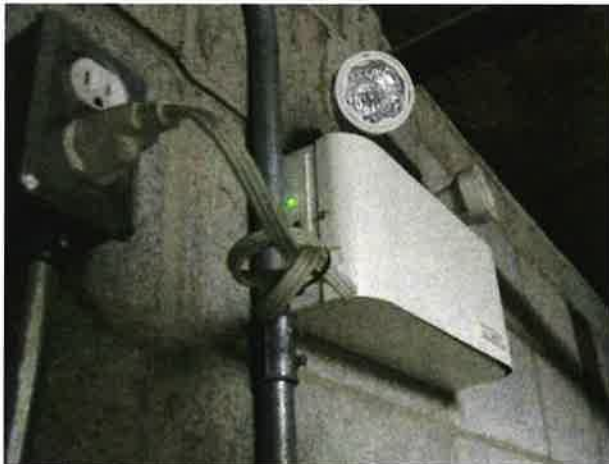
Photo 8: Emergency battery pack
