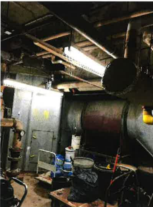
Photo 107: Water entrance, parkade exhaust, sprinkler tree, glycol pumps, and shell and tube heat exchanger
