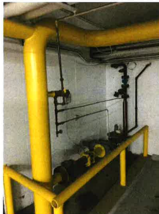
Photo 79: Natural gas meter located in parkade
