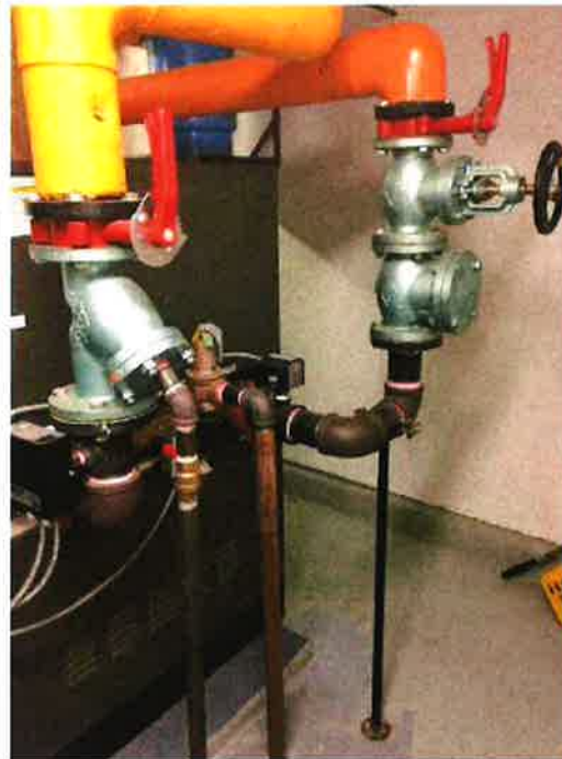
Photo 18: RBI natural gas fired heating boiler
