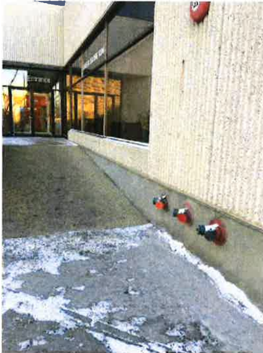
Photo 127: Fire department connections
