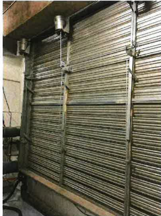
Photo 60: Penthouse supply air louvre
