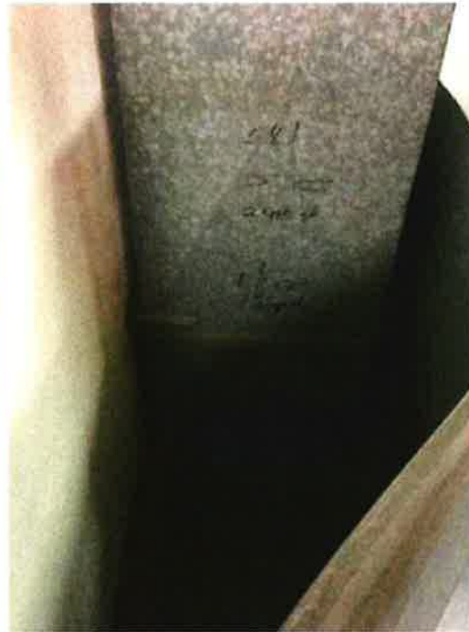
Photo 20: Fresh air intake into mechanical room, ducted down to floor with opening
