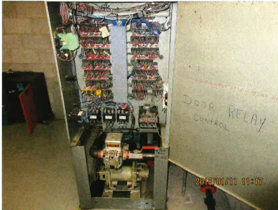
Photo 11: Controller and valve (Parkade 4)
