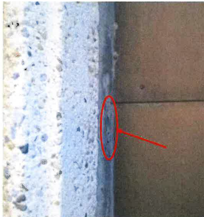
Photo 12: Deteriorated caulking at east corner of building
