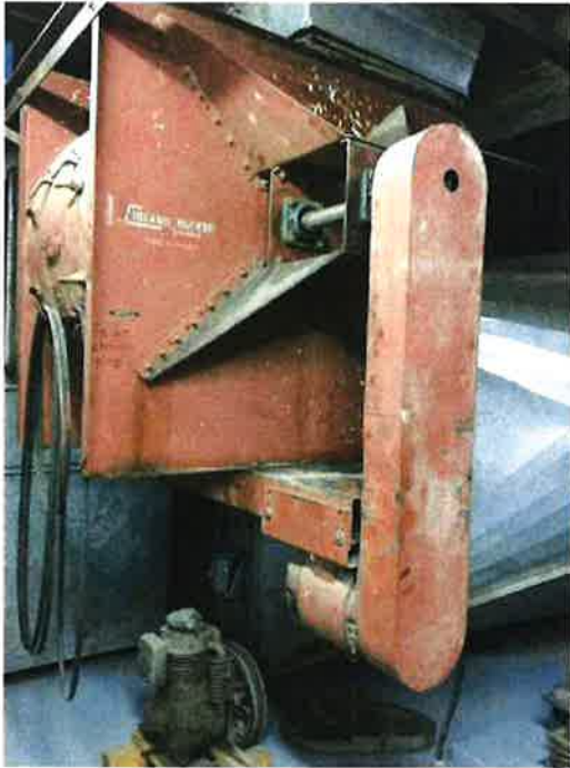
Photo 47: Central exhaust fan for washrooms
