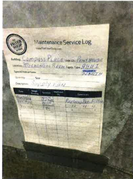
Photo 52: AHU1 supply fan service log
