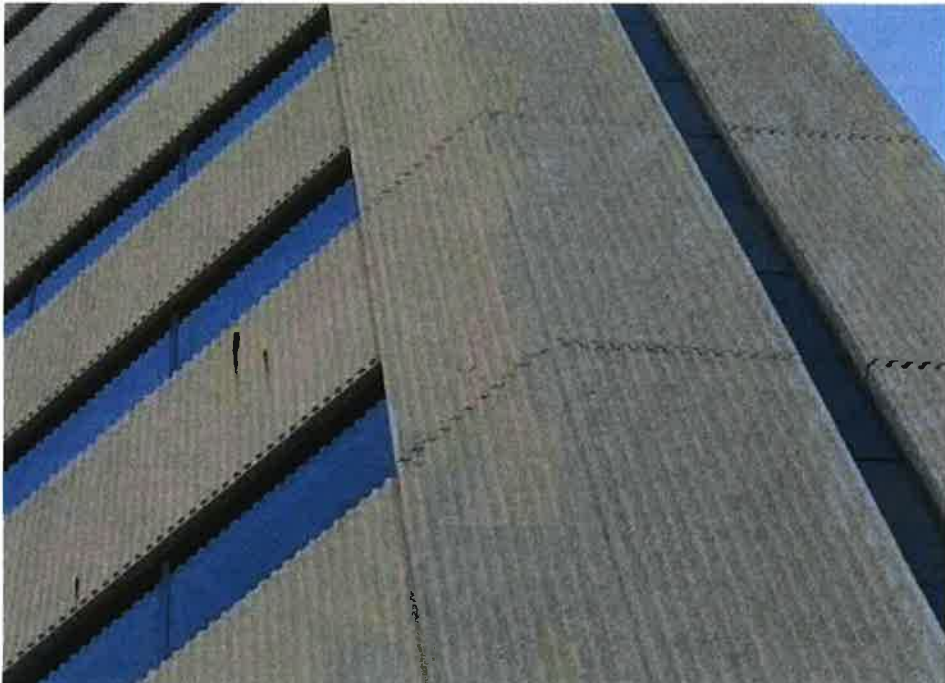
Photo 10: Stained precast on northeast elevation
