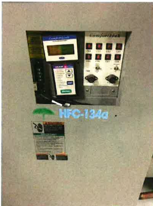
Photo 49: Chiller controls, HFC-134a Refrigerant
