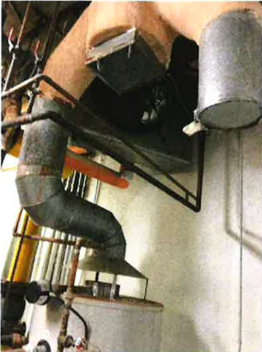
Photo 68: Domestic water heater venting
