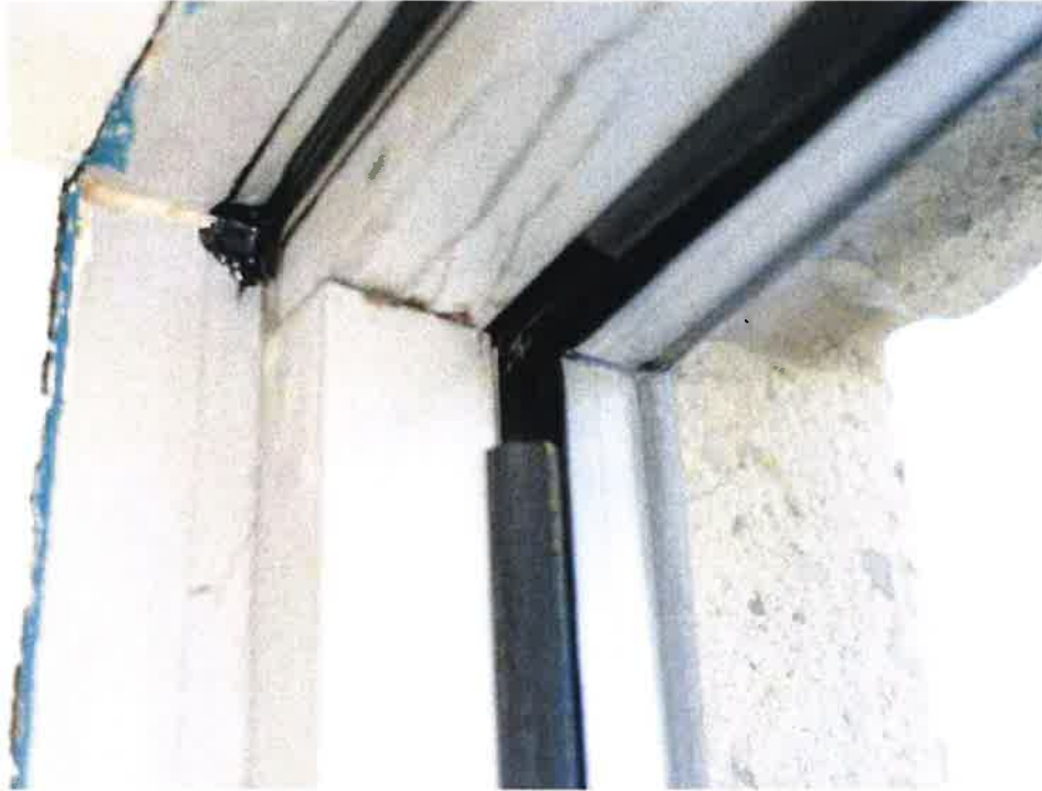
Photo 17: Shrunken gaskets on typical upper floor window
