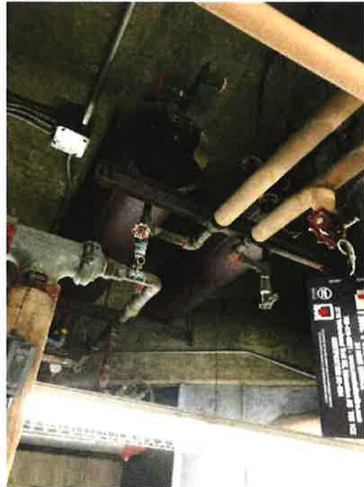
Photo 106: Expansion tanks parkade water entrance mechanical room
