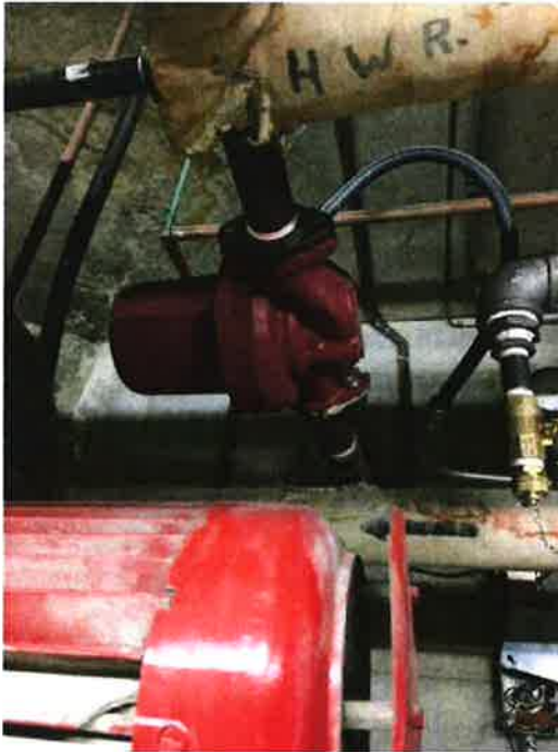
Photo 105: Hot water pump
