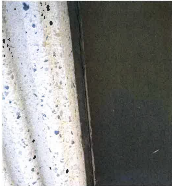
Photo 11: Failed caulking on west corner of building
