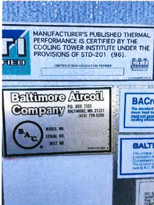
Photo 64: Cooling tower tag
