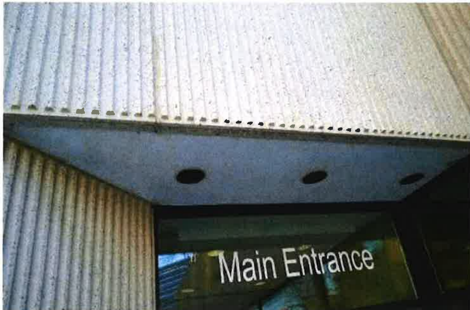
Photo 8: Stucco soffit above front entrance
