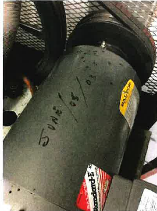
Photo 40: Air compressor motor
