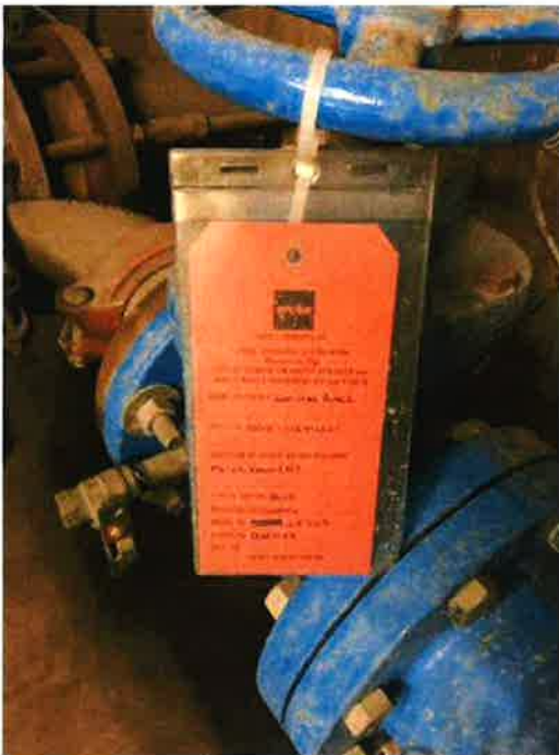
Photo 89: Double check valve assembly (DCVA) backflow preventer on domestic cold water service
