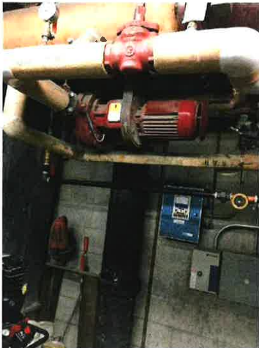
Photo 103: Glycol pump for parkade ramp snowmelt system
