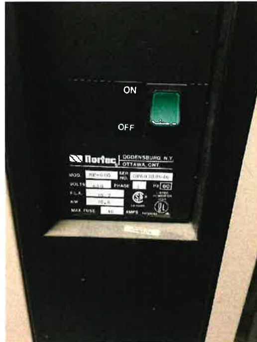
Photo 30: Typical humidifier tag for AHU1&2
