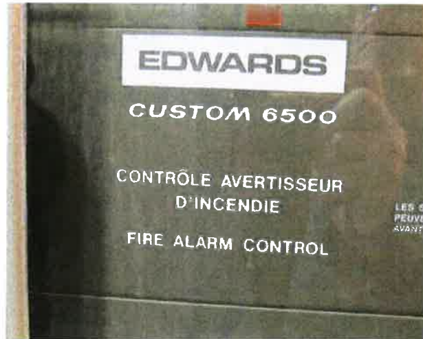
Photo 16: Fire alarm control panel 6500
