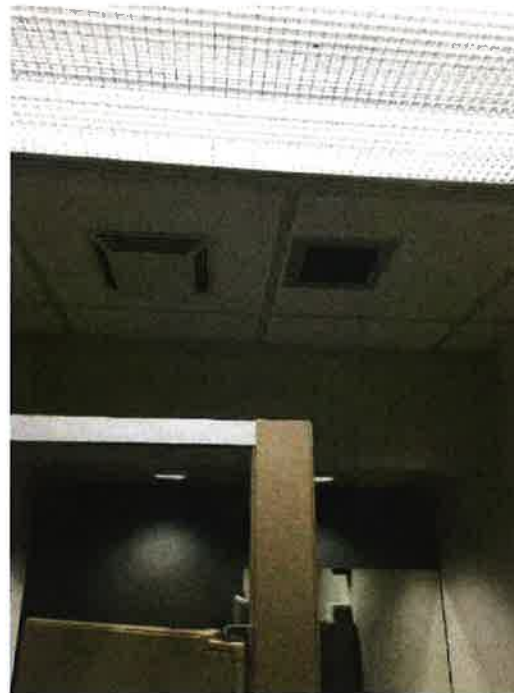
Photo 4: Washrooms have exhaust
