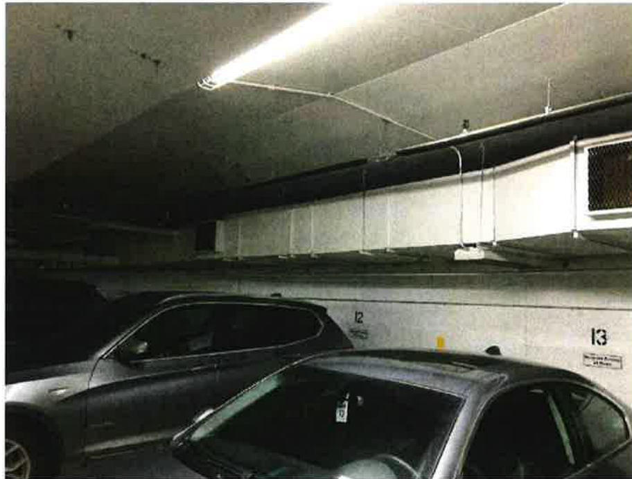
Photo 77: Typical parkade supply duct work
