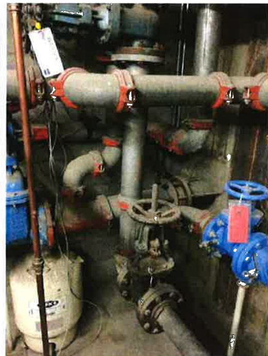
Photo 96: Fire protection incoming service
