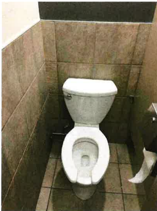
Photo 3: Typical tank type toilet
