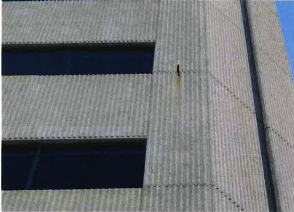
Photo 9: Stained precast on northwest elevation
