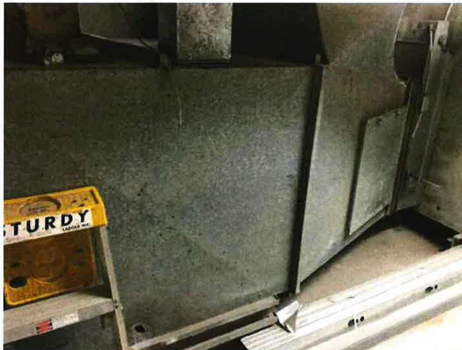
Photo 86: MAU duct work, with hole adjacent to ladder
