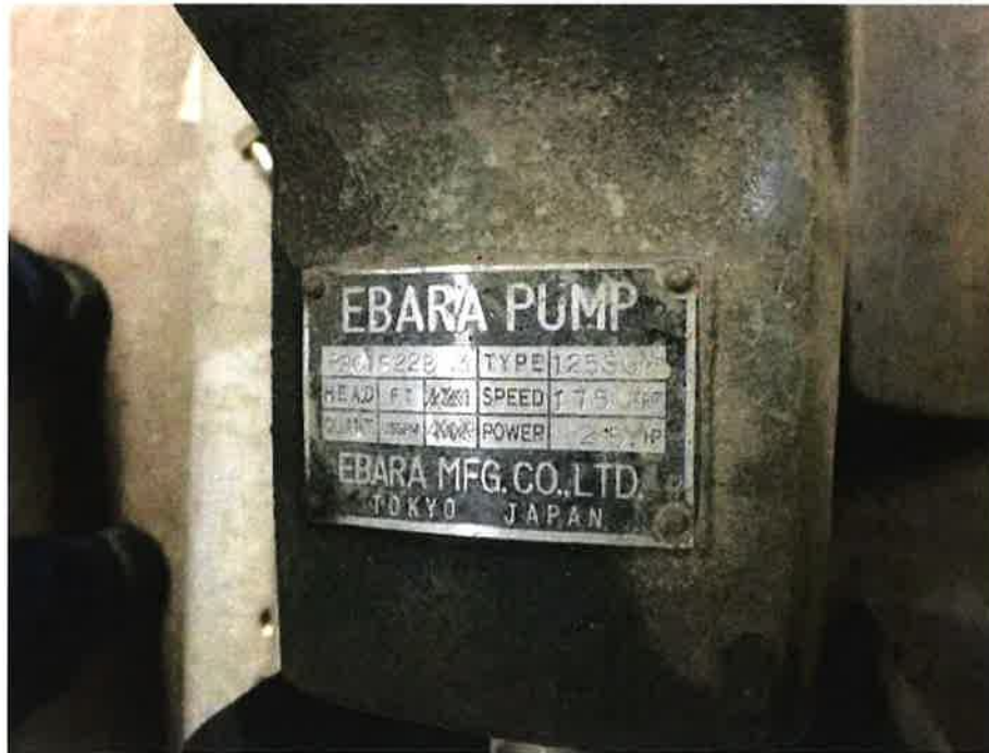
Photo 93: Secondary domestic cold water pump tag
