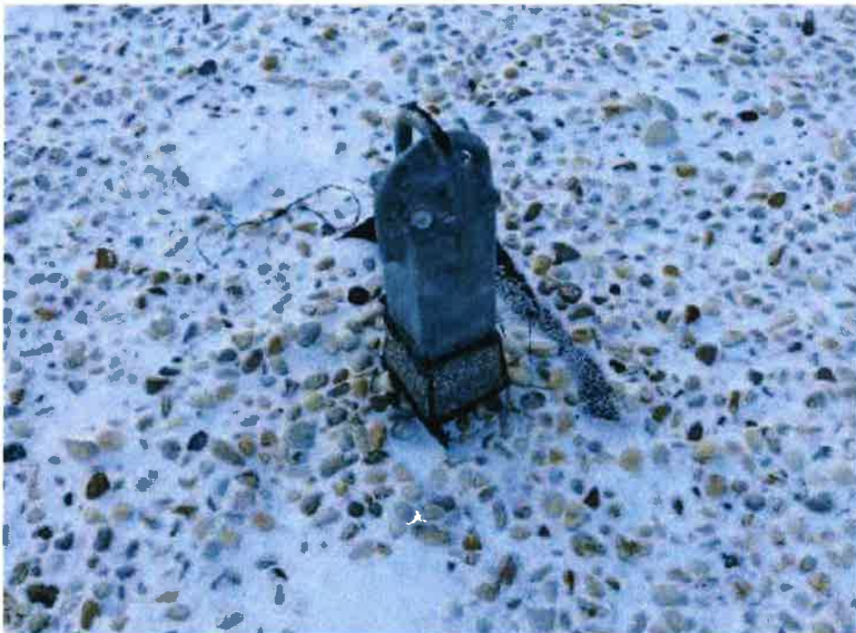
Photo 8: Exposed roof membrane at roof anchor on main tower roof
