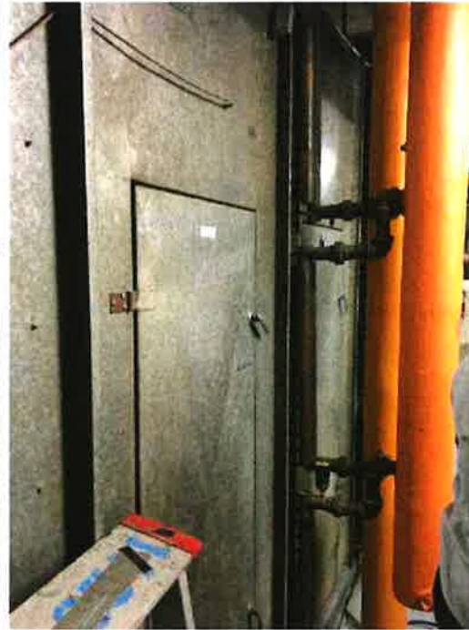
Photo 32: Heating coil for 'AHU2'
