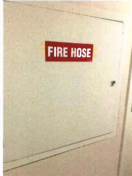
Photo 75: Fire hose cabinet
