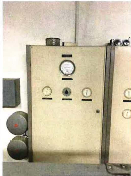
Photo 36: Honeywell control panel for AHU2 (Control CCT 33, Panel A) Part 1
