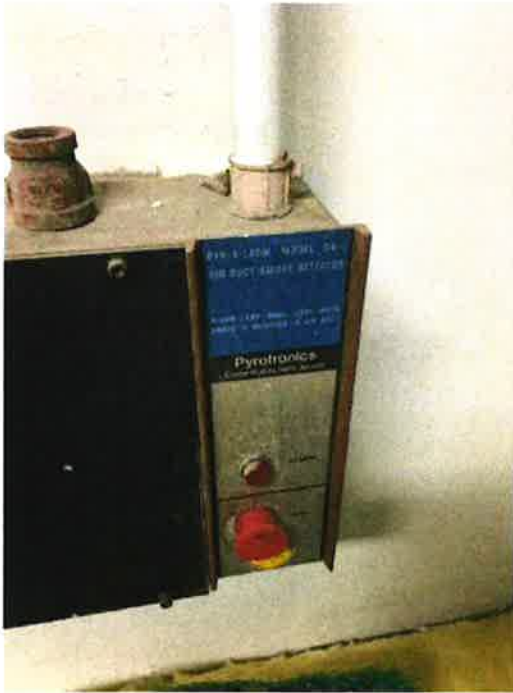
Photo 66: Air duct smoke detector alarm panel
