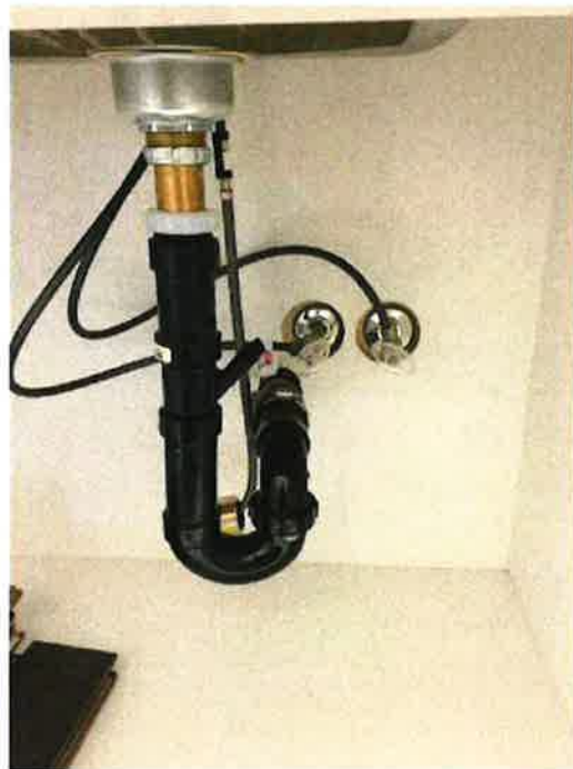
Photo 73: Typical tenant plumbing below sink
