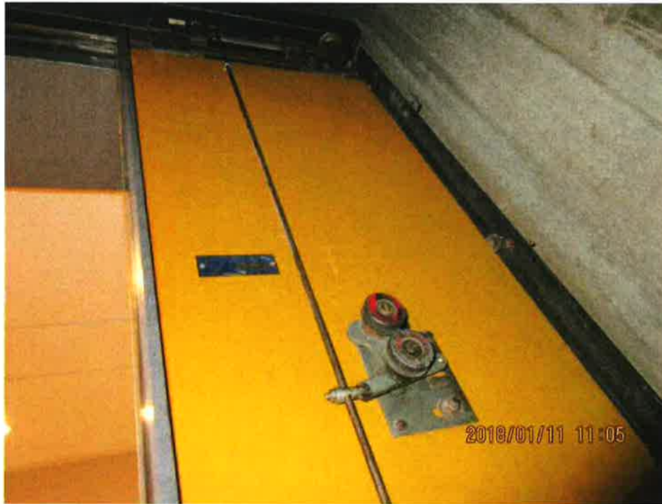
Photo 5: Typical hall interlock assembly (Passenger 1-3)
