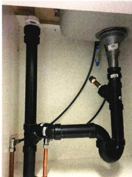
Photo 76: Tenant sink with an air admittance valve
