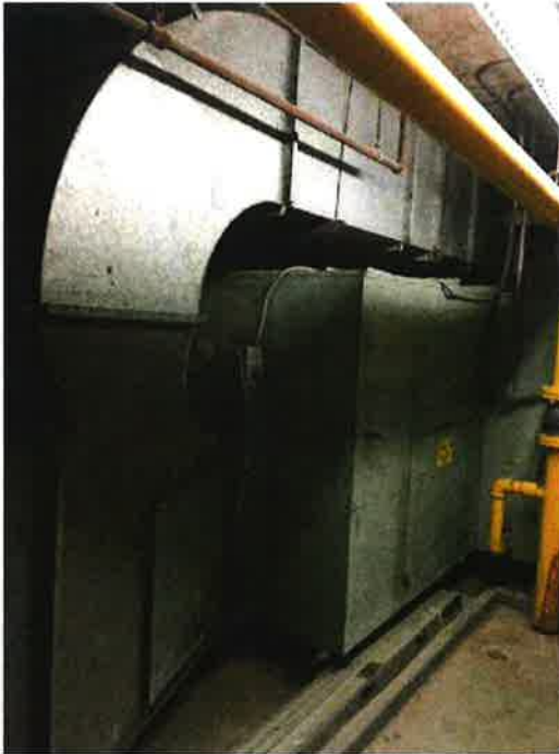
Photo 87: MAU and duct work
