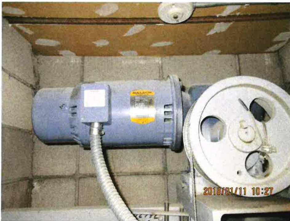
Photo 18: Hoist machine (Dumbwaiter 5)
