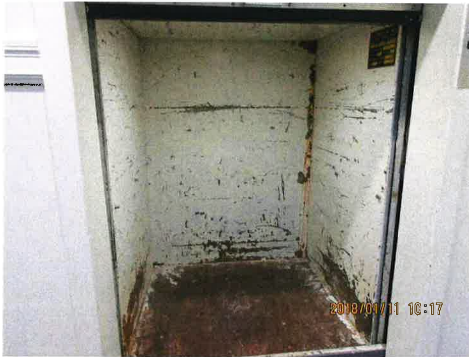
Photo 21: Cab interior (Dumbwaiter 5)
