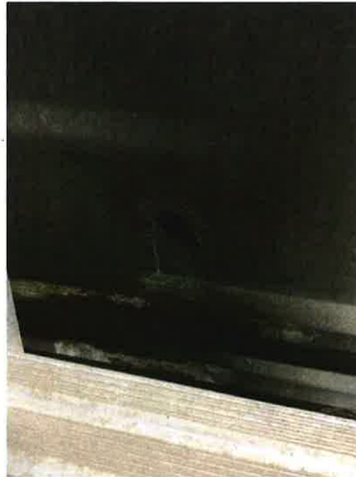
Photo 85: Hole in side of MAU supply ductwork
