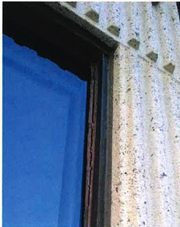
Photo 14: Failed caulking at typical glazing joint
