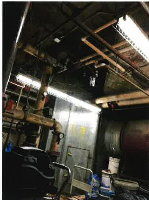
Photo 108: Parkade mechanical room piping
