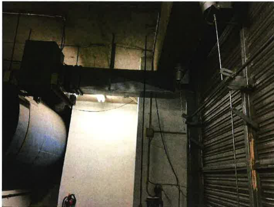
Photo 61: Fan adjacent to intake louvre
