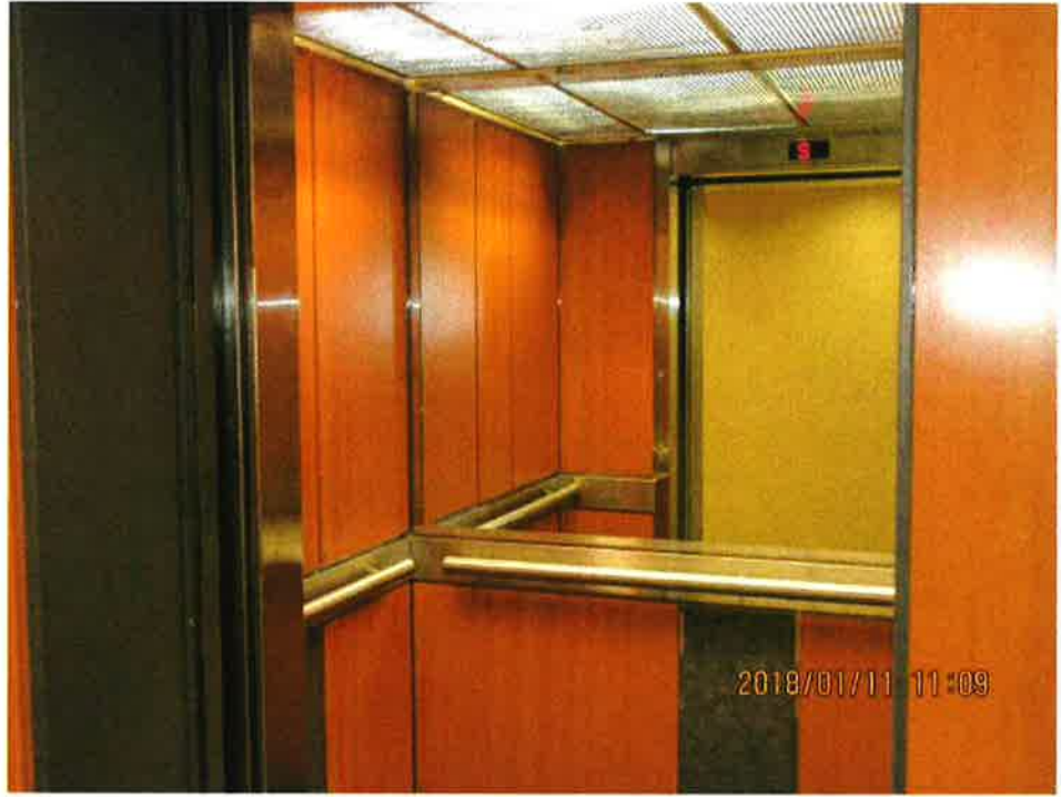
Photo 7: Typical cab interior finishes (Passenger 1-3)
