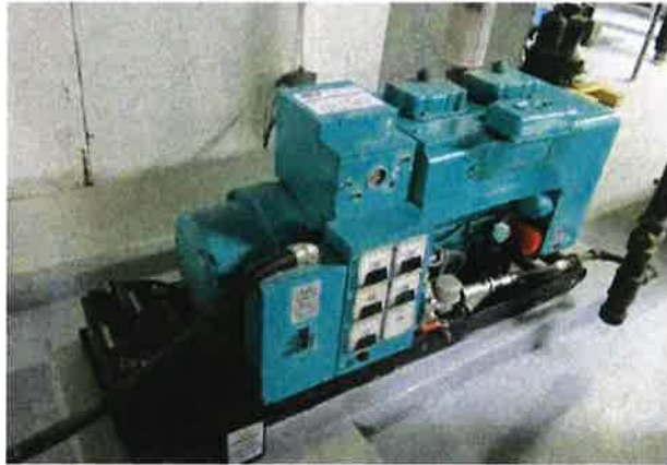
Photo 13: Gaseous emergency generator
