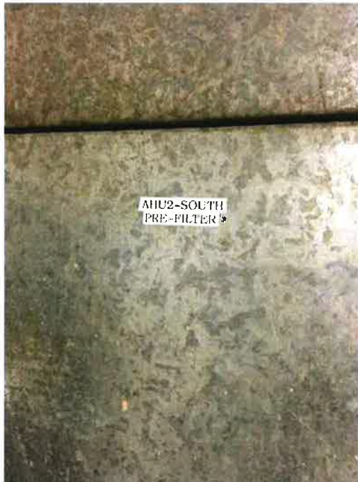
Photo 35: AHU2 has a pre-filter
