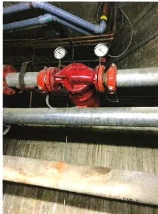
Photo 98: Fire pump, missing pipe support on right hand side.
