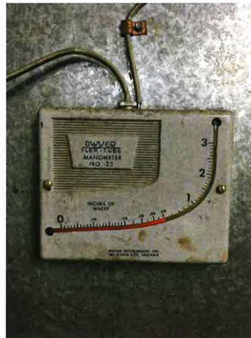
Photo 34: Differential pressure gauge around filter on AHU2
