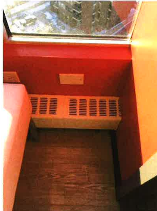
Photo 6: Typical perimeter hydronic heating
