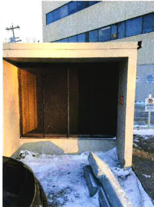
Photo 124: Parkade MAU outdoor air intake
