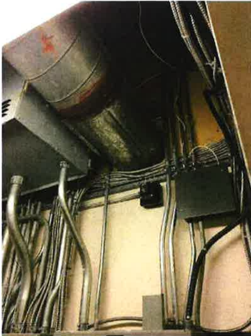
Photo 70: Typical electrical room grille above spiral duct for electrical room ventilation
