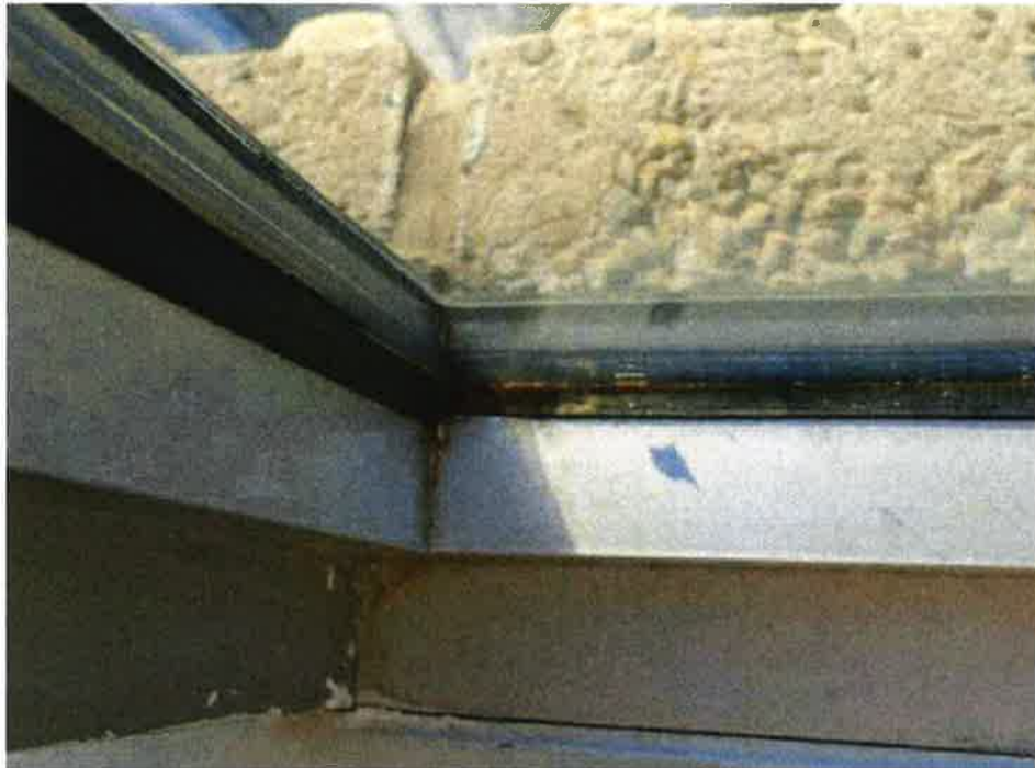
Photo 18: Stains at bottom corner of typical upper floor window
