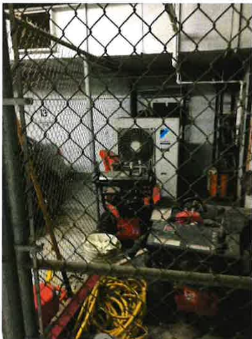
Photo 78: Condenser located in parkade
