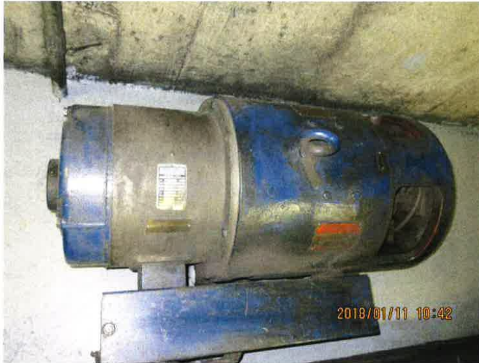
Photo 3: Typical motor-generator (M-G) set (Passenger 1-3)
