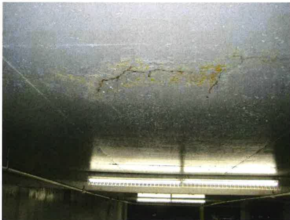
Photo 6: Active leak location below entrance/exit ramp
