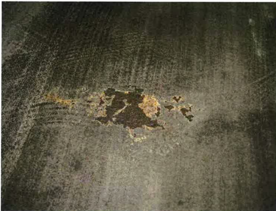
Photo 8: Typical coating wear, exposing concrete surface below
