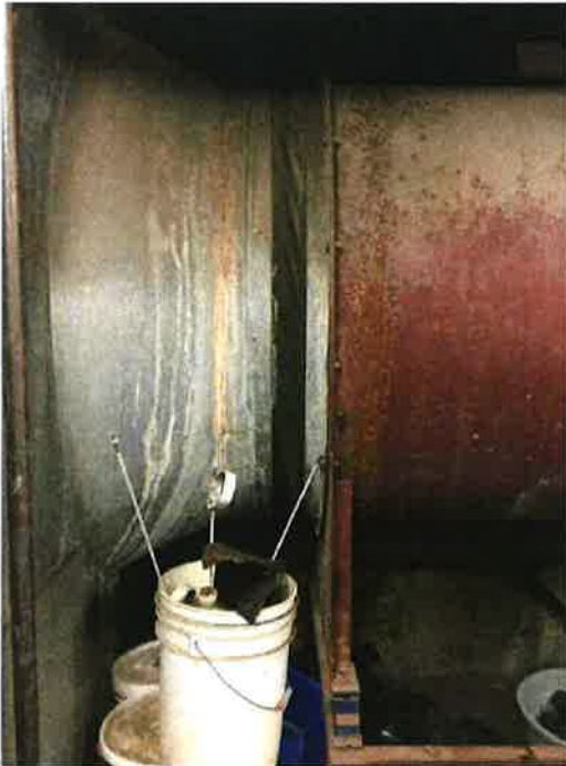
Photo 101: Parkade exhaust fan outlet connection to exhaust air plenum showing signs of rust
