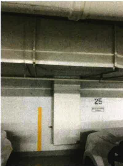
Photo 82: Parkade exhaust duct work on opposite side from supply. Open ended duct at low level.
