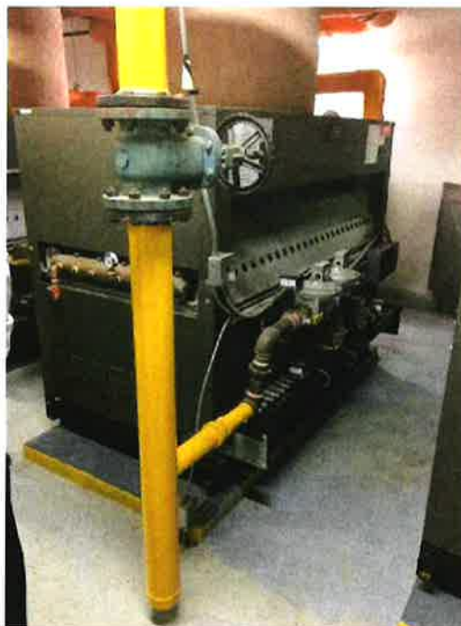
Photo 14: RBI natural gas heating boiler
