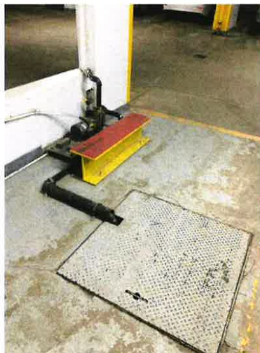
Photo 114: Parkade sump pump and pit
