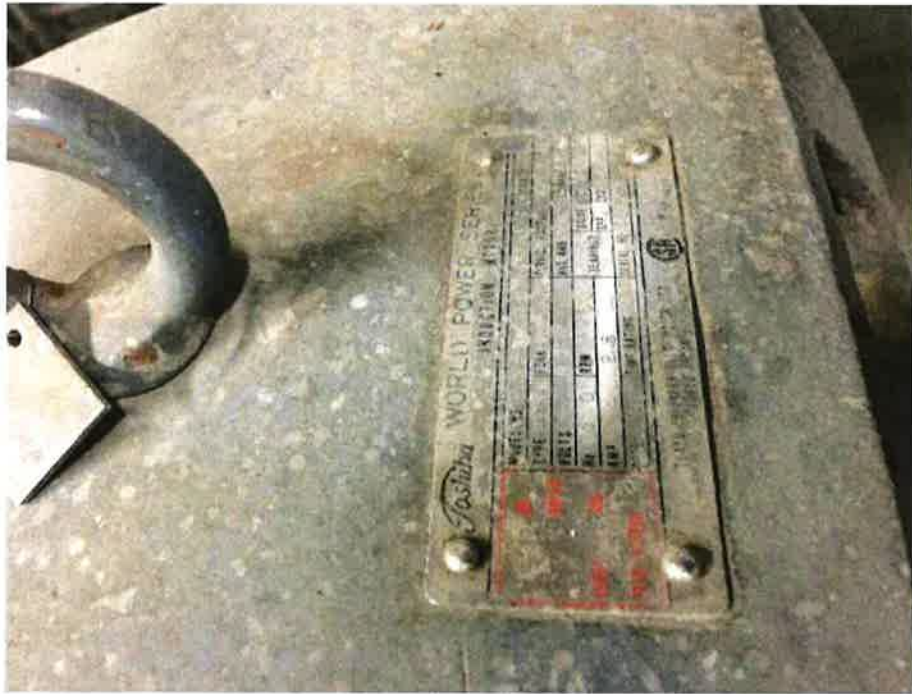
Photo 94: Secondary domestic cold water pump motor tag
