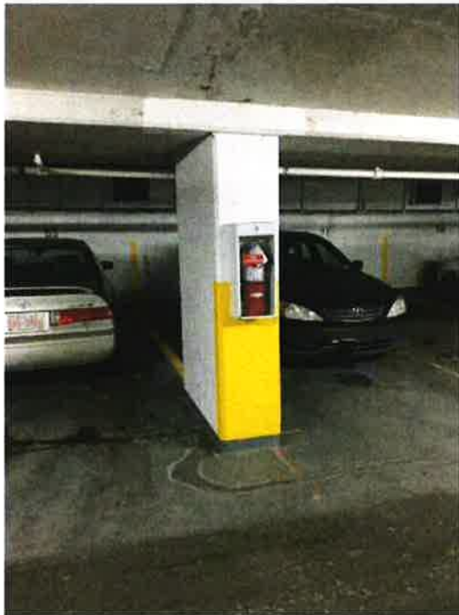
Photo 111: Sprinklers and fire extinguishers throughout parkade
