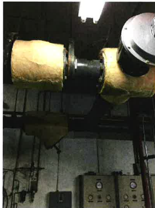
Photo 42: Chilled water piping and insulation (showing mold growth)
