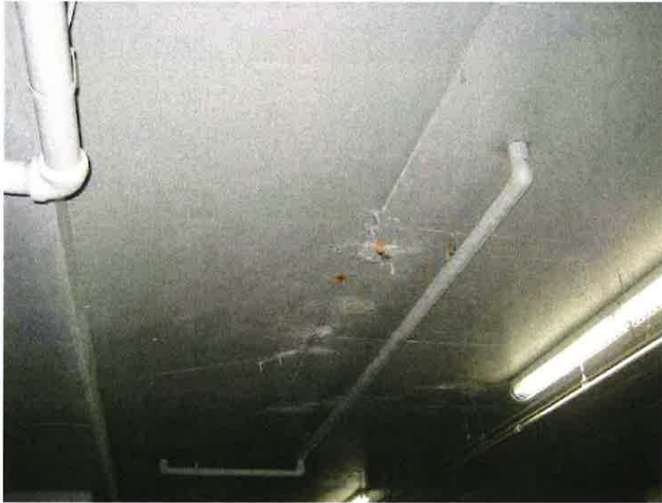
Photo 5: Typical staining below suspended parking level
